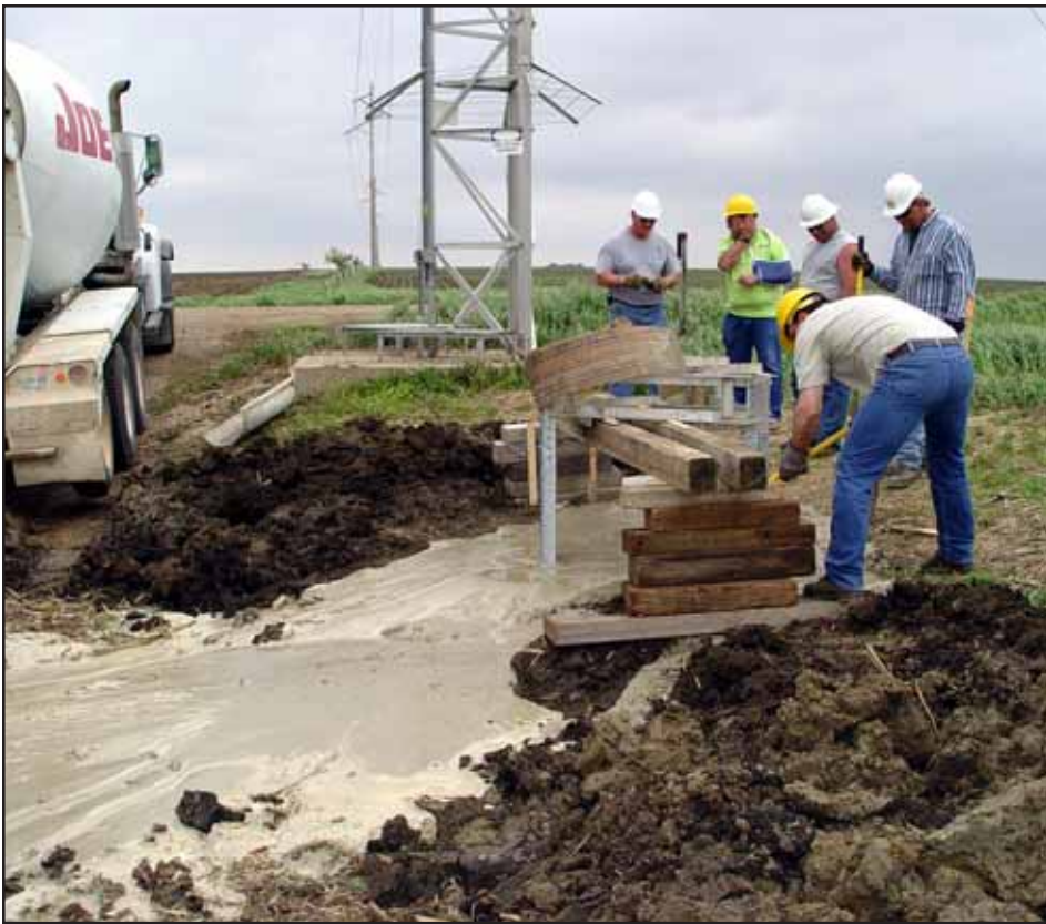
NIPCO's crew pours a new concrete pad prior to moving switch tower K223 27 feet west to allow for a Sioux County road widening project.
