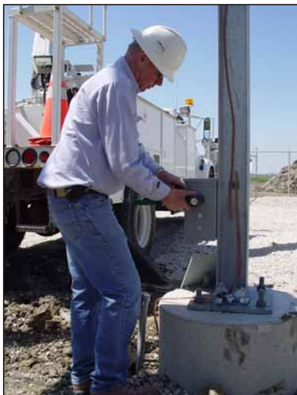
Jerry Lubben, electrician foreman, pulls a cable to a control panel at the enlarged Galva Substation.
