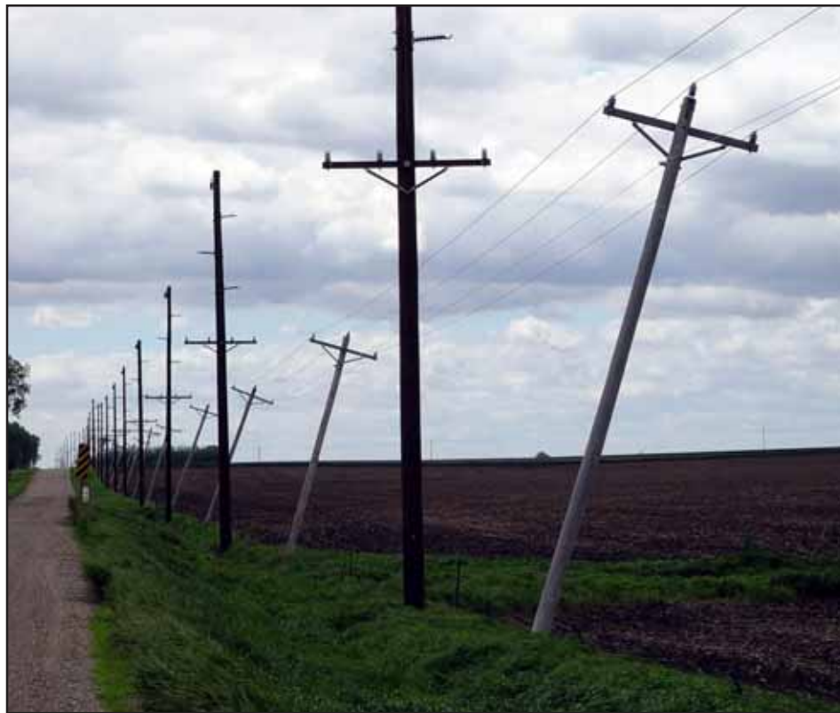
New poles have been set for NIPCO's 69-kV line to bypass the town of Sioux Center. Existing poles were leaned over to make room for the new poles.
