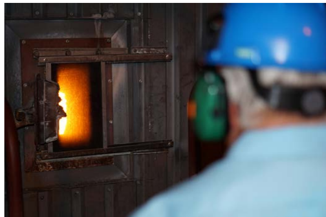
Tour participants get a peek into the 277' tall boiler at Antelope Valley Station.
